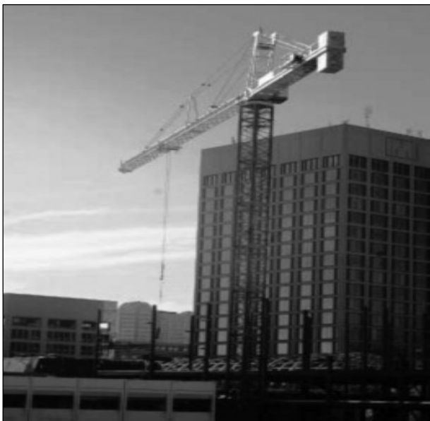
OE DAVE DOBSON AND 4 TH YEAR APPRENTICE TOM MCEVOY SETTING IRON FOR UNIVERSAL STEEL AT THE CITY SQUARE PROJECT IN WORCESTER
