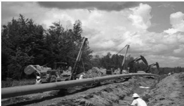
Schmid Pipeline Construction and members of the Operating Engineers Local 4 laying 30" pipe from the St. Croix River to the Baileyville Compressor Station in Washington County, Maine for Maritimes Northeast Phase IV project.
