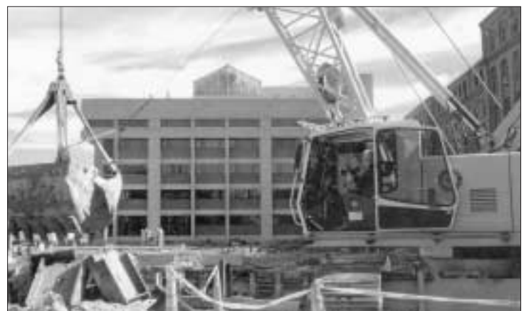
Local 4 Operator Jim Black is working at Harvard University in Cambridge for J.F. White.
