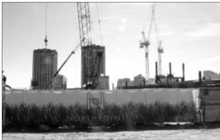
North Point Park, Cambridge Capco is setting steel with the help of their two tower cranes. Builders Resource Inc. is setting steel on another building as this project goes forward.
