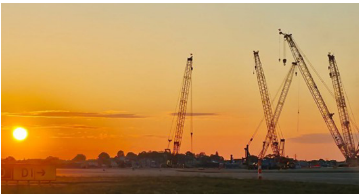
J.F. White driving piles for McCourt's runway extension project at Logan Airport.
